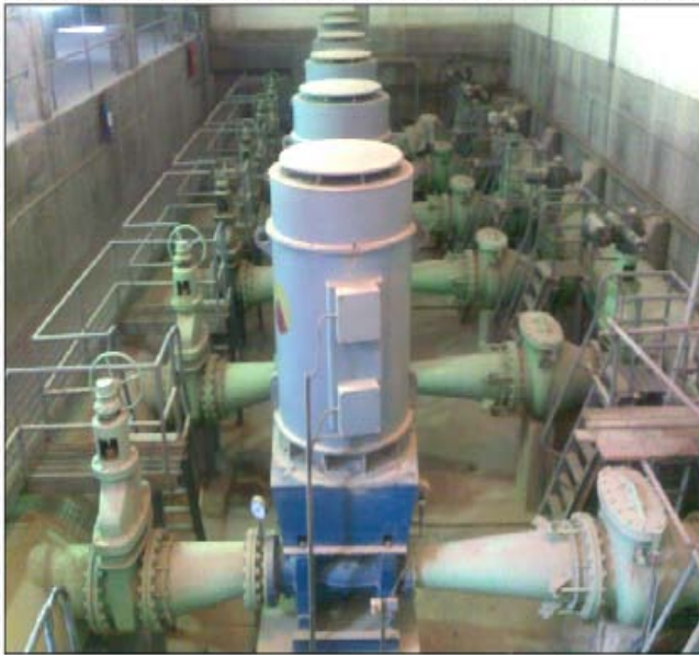
A. Pumps in NPS-1
