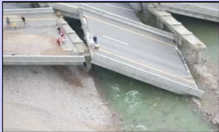
Road Destruction in Muscat
