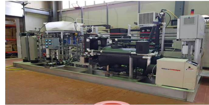
FO Pilot Test Plant
