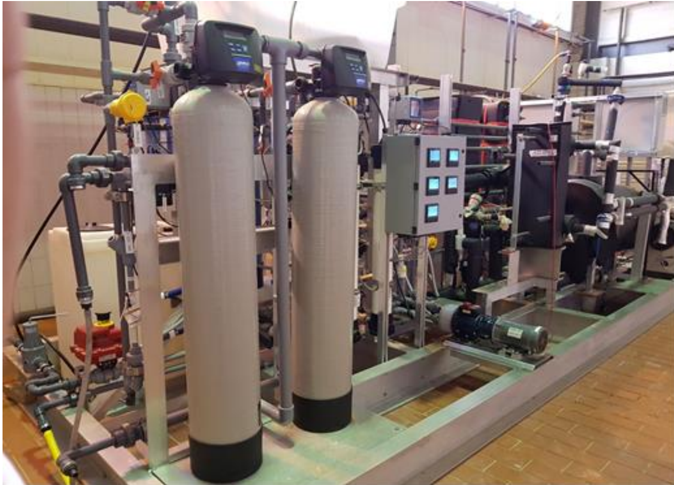
Post-treatment unit of FO Pilot Plant Test Unit
