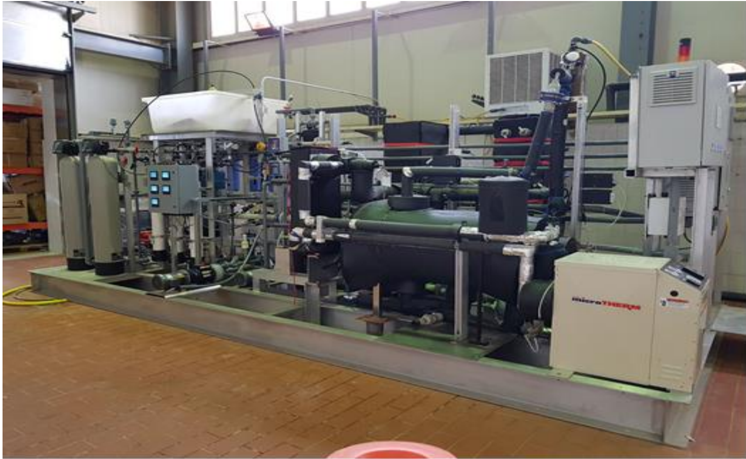
FO Pilot Plant Test Unit with a Capacity of 10 m 3 /d
