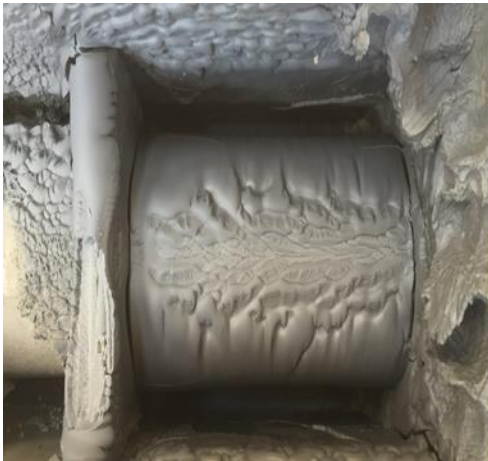
Heat exchanger covered with silt
