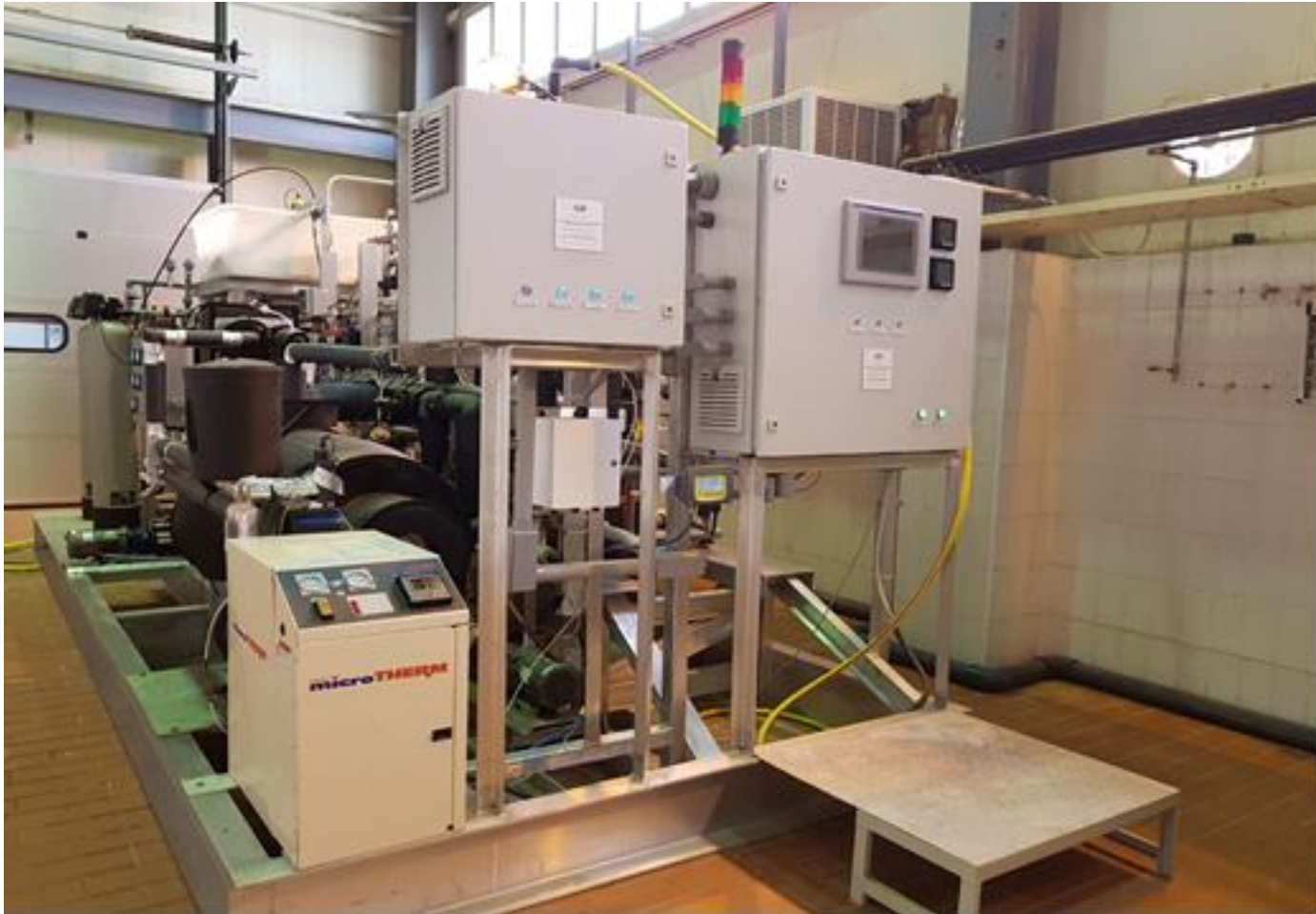
Control and Data Acquisition System
