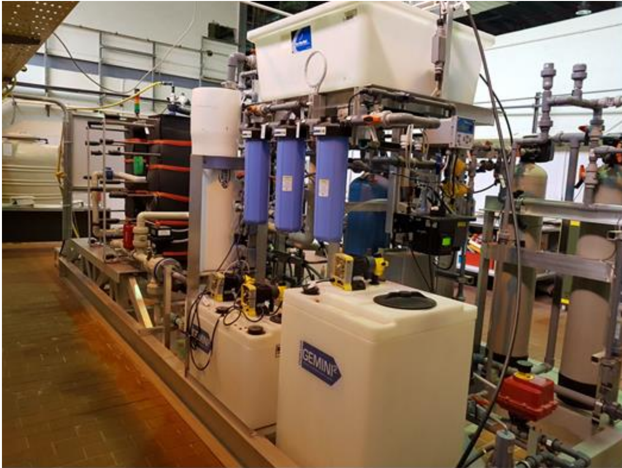
Pre-treatment unit of FO Pilot Plant Test Unit
