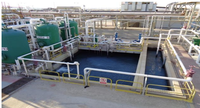
Wastewater Treatment Plant at Gulf Petrochemical Industries Company (GPIC)/ Wastewater generated by economic activities. Curtesy GPIC
