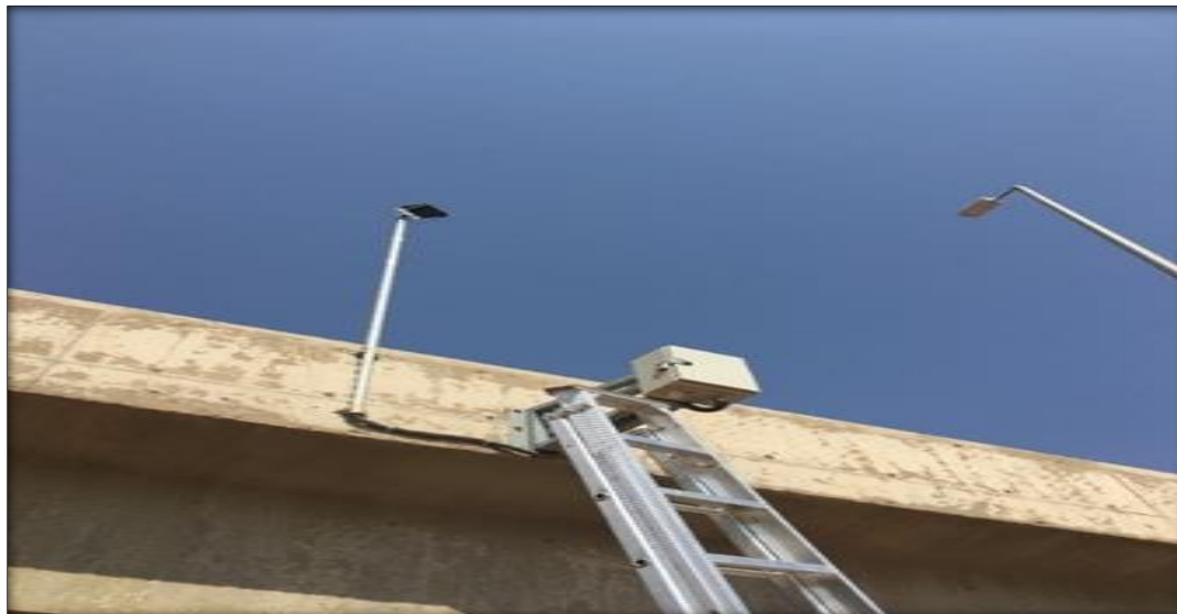
MEWA hydrologic network Runoff station.
