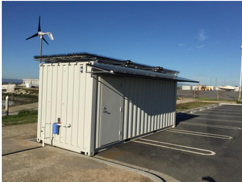
Image of Test Unit with a Plant Capacity of 50 m 3 per day
