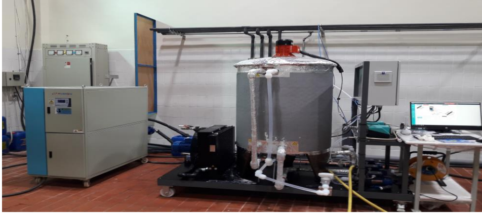
Image of Pilot crystallization test unit installed at KISR site
