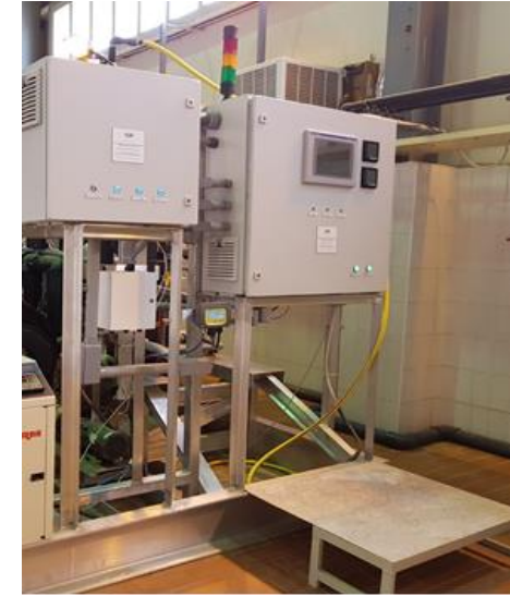
Control & Data Acquisition Systems
