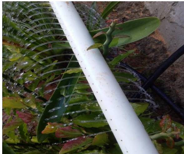
Figure 4. Permeate tube for irrigation
