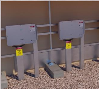
Solar PV Inverters
