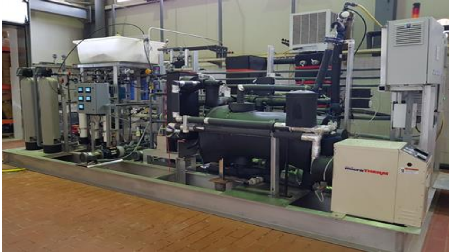
Investigated FO Pilot Plant Test Unit at KISR
