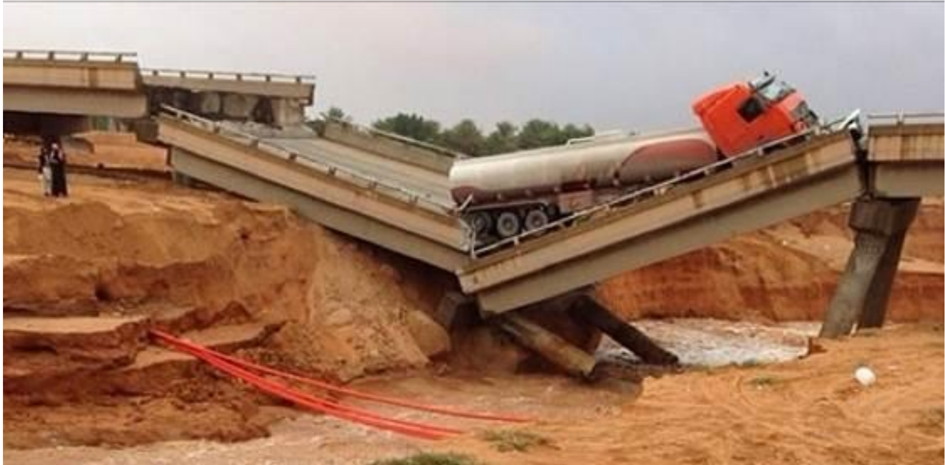
Figure (1) : The Failure part in Thomam Bridge
