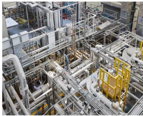
The small pilot plant, which uses solar energy to heat the water for desalination.
