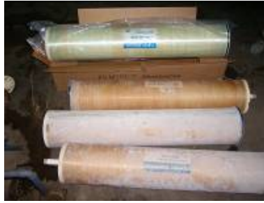
Figure 4: Membranes condition during the year of 2006.
