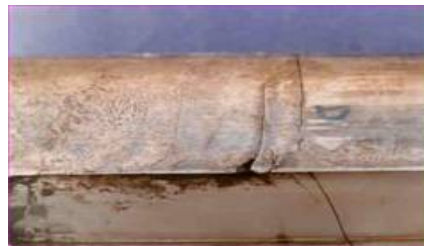
Figure 2. Section of the Shaft showing the cracks. Corrosion is seen on the key slot surface and on the corners
