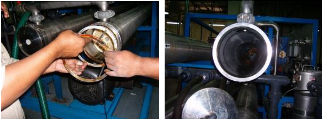
Figure 5: Original stainless steel vessel and new replacement
