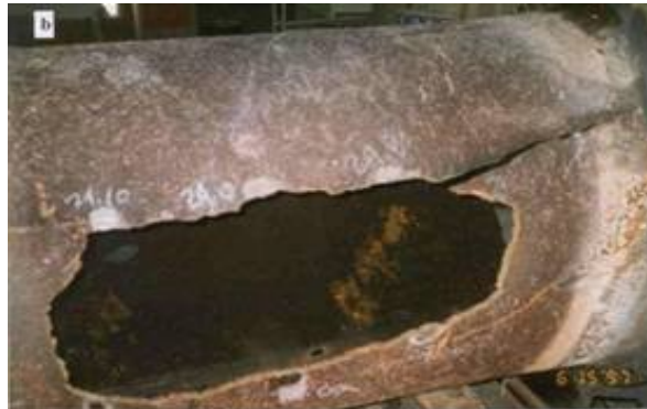
Figure 7. Close view of the damaged column pipe showing crack extending up to the end of the flange
