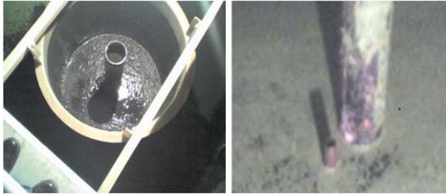
Figure 7: View of the Clarifier Tank. Figure 8: View of the pipe after removing
