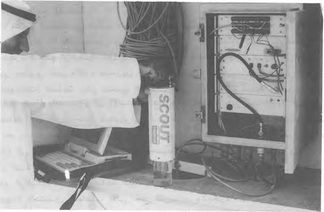
Figure 2. Operational Data Collection Platform near Al Ain.
