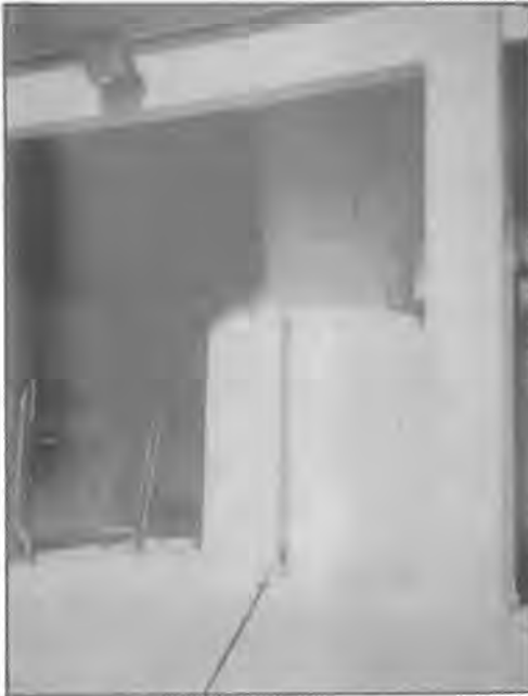
Fig. 4. Alkali storage tank leaking at the bottom.
