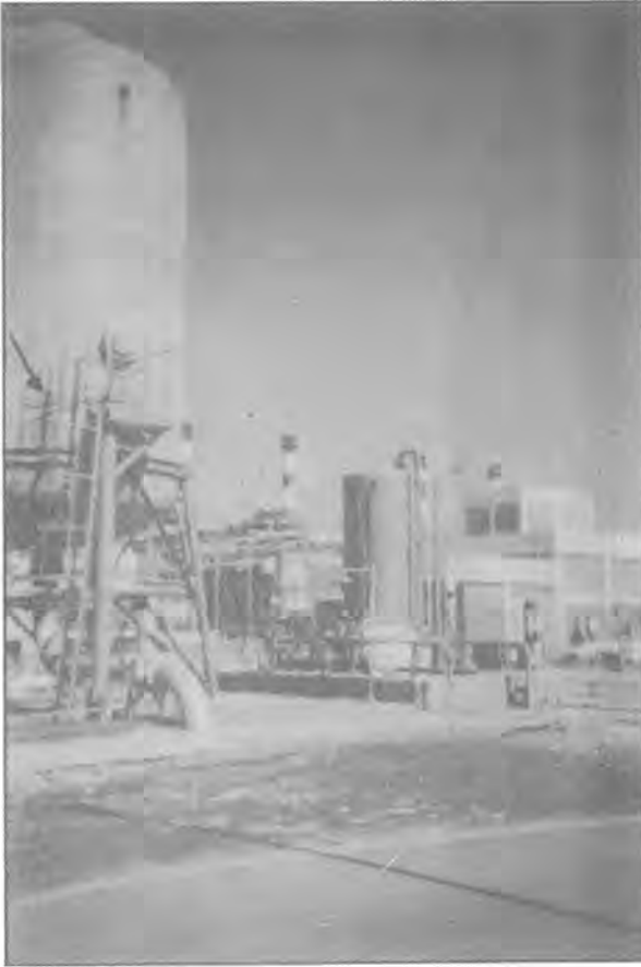
Fig. 3. Hypochlorite tank with leak near manhole.
