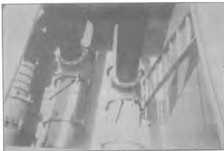
Fig. 2. The injection point with new spools inside a concrete pit
