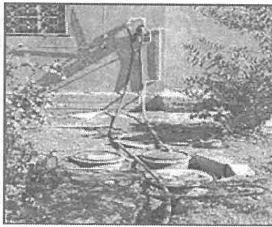
Figure 1: Four-Barrel Greywater Treatment Unit
